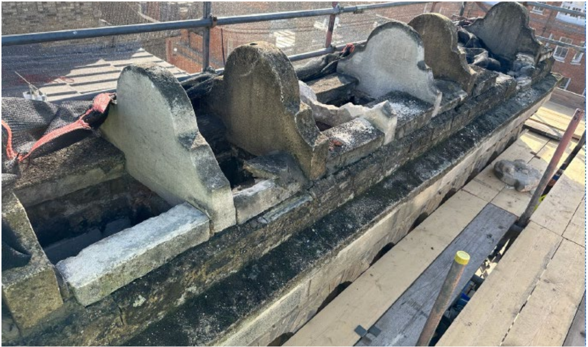
Overview of the wrapped section of the end slack before rebuilding works commenced.
