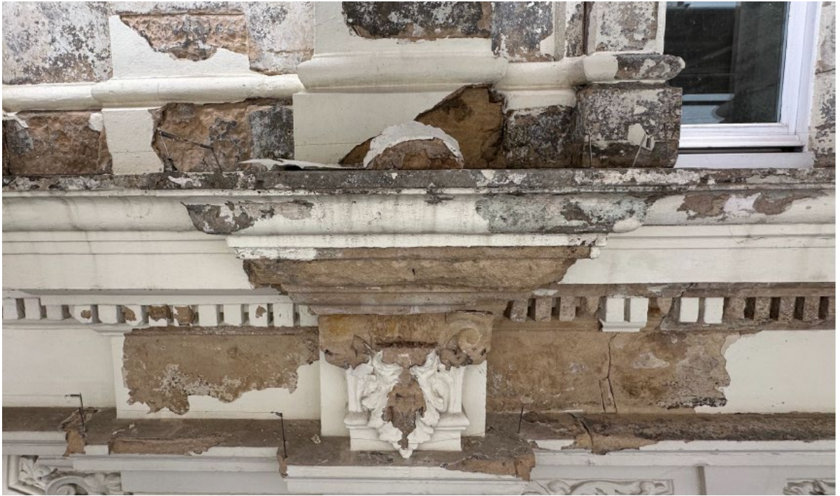
Extent of Bath Stone Repairs required, before works commenced.
